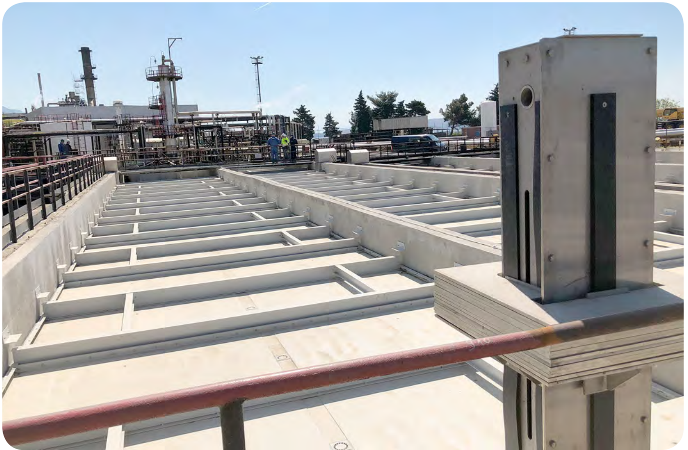
API tanks with floating GRP covers
