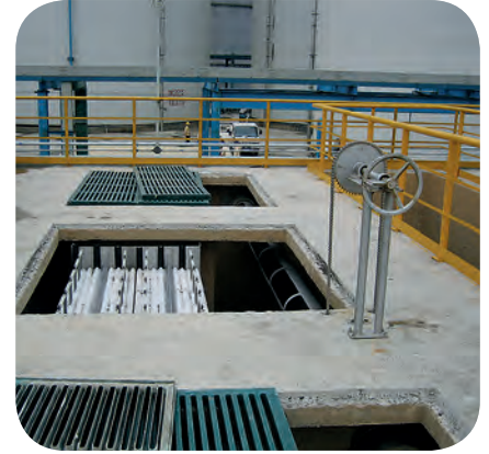
CPI installations with covers
