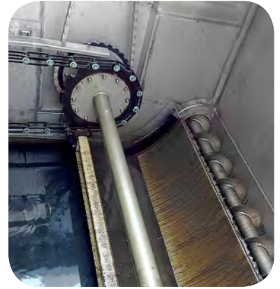
DAF scraper with sludge removal using a ramp and screw conveyor
