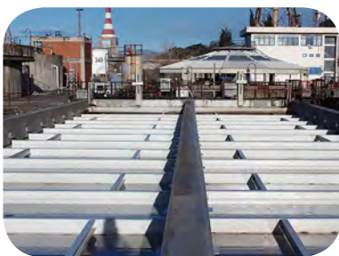
API tanks with floating GRP covers
