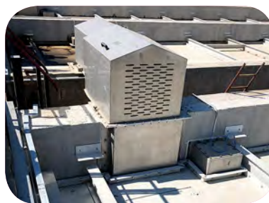
API tanks, gas-tight
